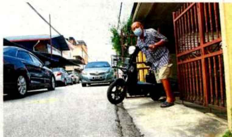
Wong showing the raised edge of the road that is higher than his house porch. — CHAN TAK KONG/The Star
